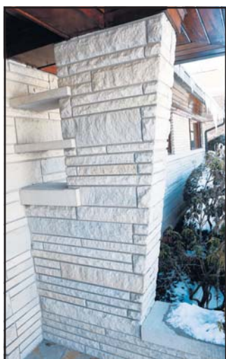
Part of the entry in the Ernst Johnson designed home on Ashwood Drive.
