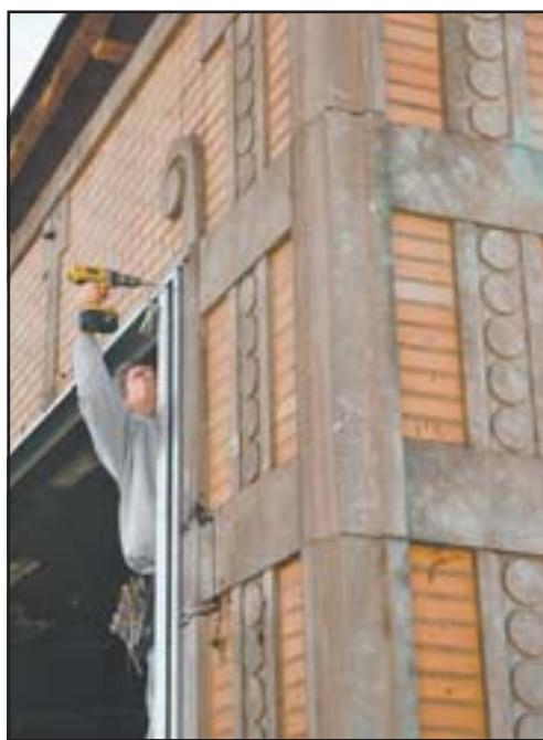
Steve Sparks of Angelucci Acoustical Inc. installed metal framing for a cement board Tuesday at the East Main buildings.
